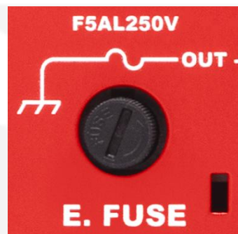
Figure 28: Earth fuse housing.
