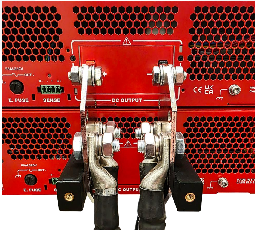
2.5Figure 37: Load cables connection
